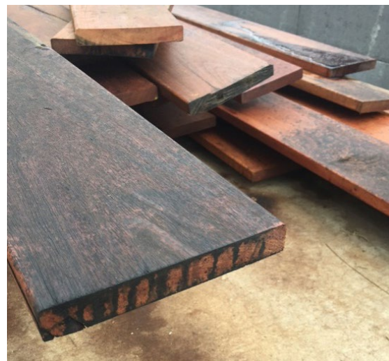
Photograph 2 - Mould stains on linseed oiled decking
